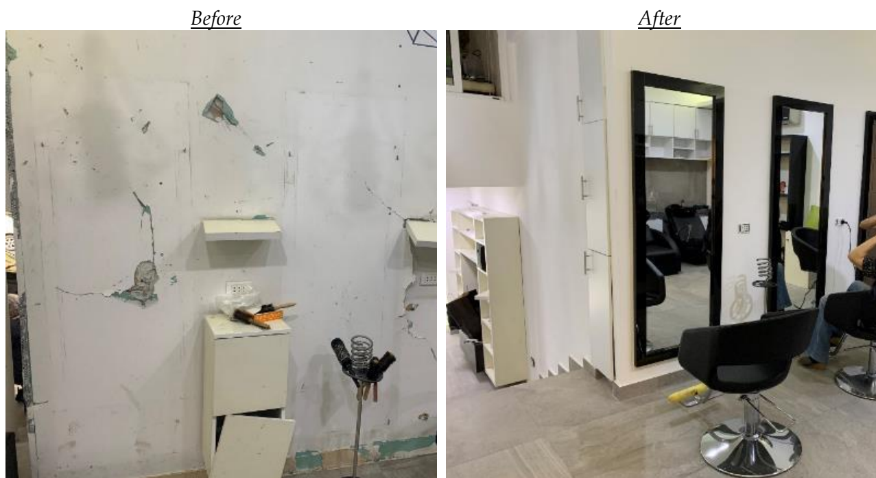
Before and after repairs to a hair salon in Ashrafieh, which included the installation of new gypsum board walls, painting, and providing new salon chairs and mirrors.
