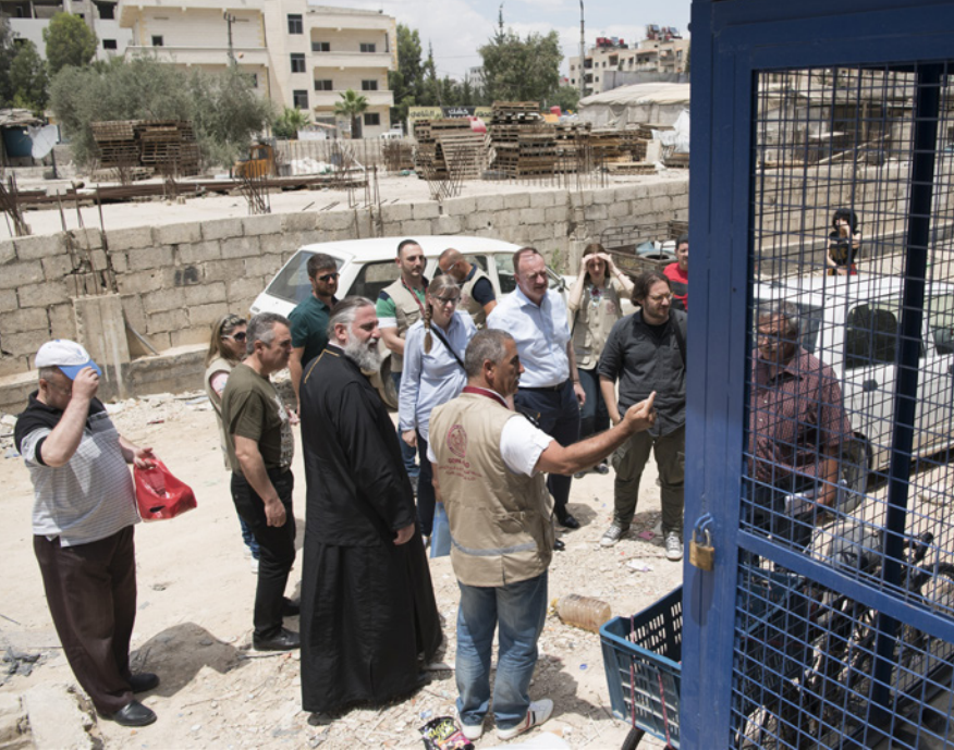
SYRIA, DAMASCUS, 2018: Renovation of urban water infrastructure in the Jaraman neighbourhood, with appropriate security fencing. Father Alexis of the Greek Orthodox Church is accompanying a visiting delegation from NCA. Father Alexis headed the diaconal aid agency of the church until he tragically died from a Covid-19 infection during the height of the pandemic. (Photo: Håvard Bjelland/NCA)
