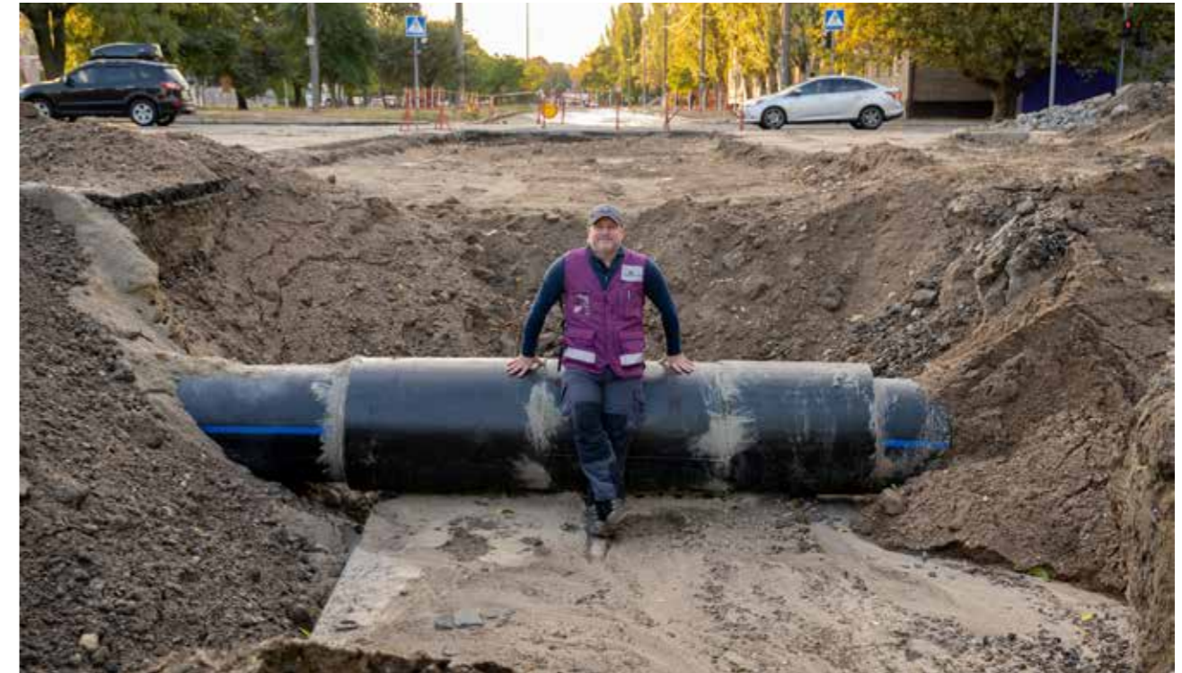
WASH Coordinator Damian Seal at the pipe that supplies heating to 160,000 people in Mykolaiv, Ukraine. Photo: Håvard Bjelland/Norwegian Church Aid
